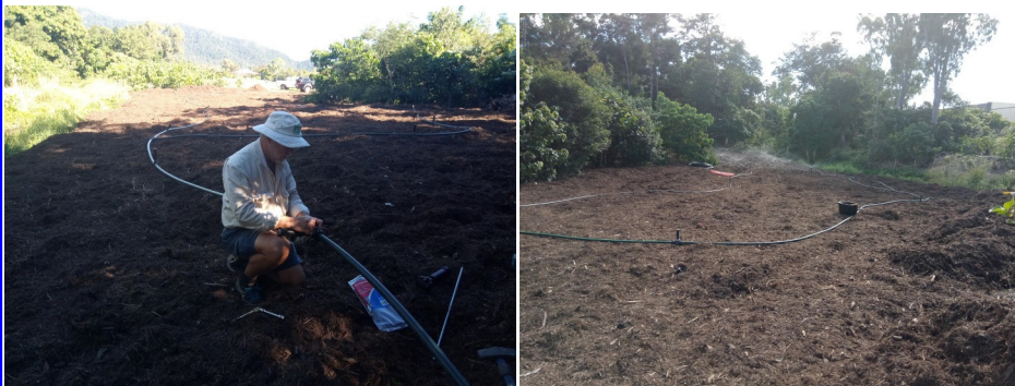
Above: Jim installing the irrigation & then it all set up & pre-watering before planting on Sunday. Photo: Dave Young
